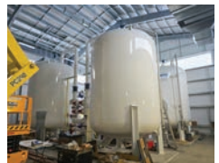
EAST STREET WTP/PFAS FILTRATION SYSTEM - VESSELS JANUARY 2026
