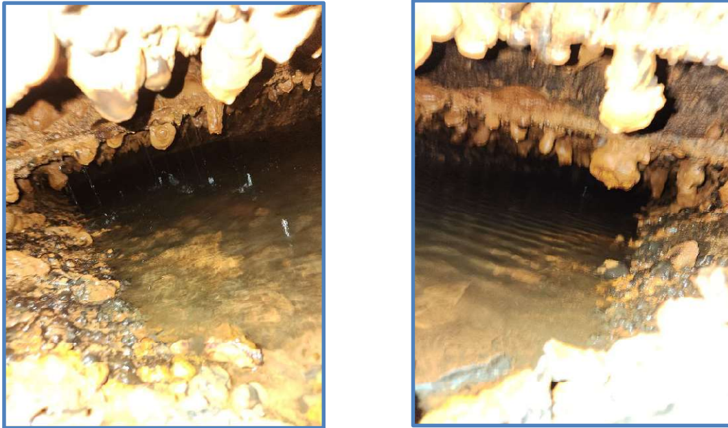
Figure 4/5: Underdrain plenum looking to the left and right from the manway opening of Filter 1
