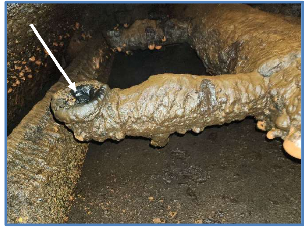
Figure 1: 1 of 8, 3" inlet distributors in Filter 1, Cell A
